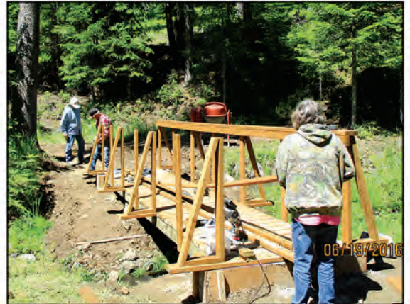
Lions Cheri Jackson, Bruce Bugbee and Cliff Storey working on the bridge
