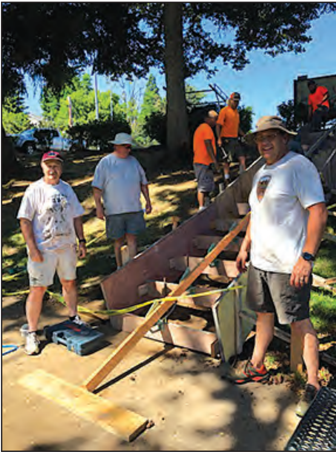
The stairway under construction. (l-r): Lions Mike Schend (chairman of the project), Greg Simpson and Jess Flem. The guys behind in orange are construction workers.
